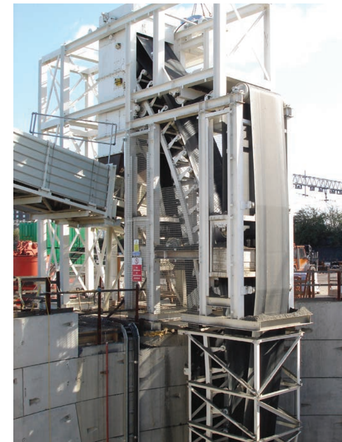
The HAC system is a proven method for conveying materials vertically from tunnelling operations to the surface.
